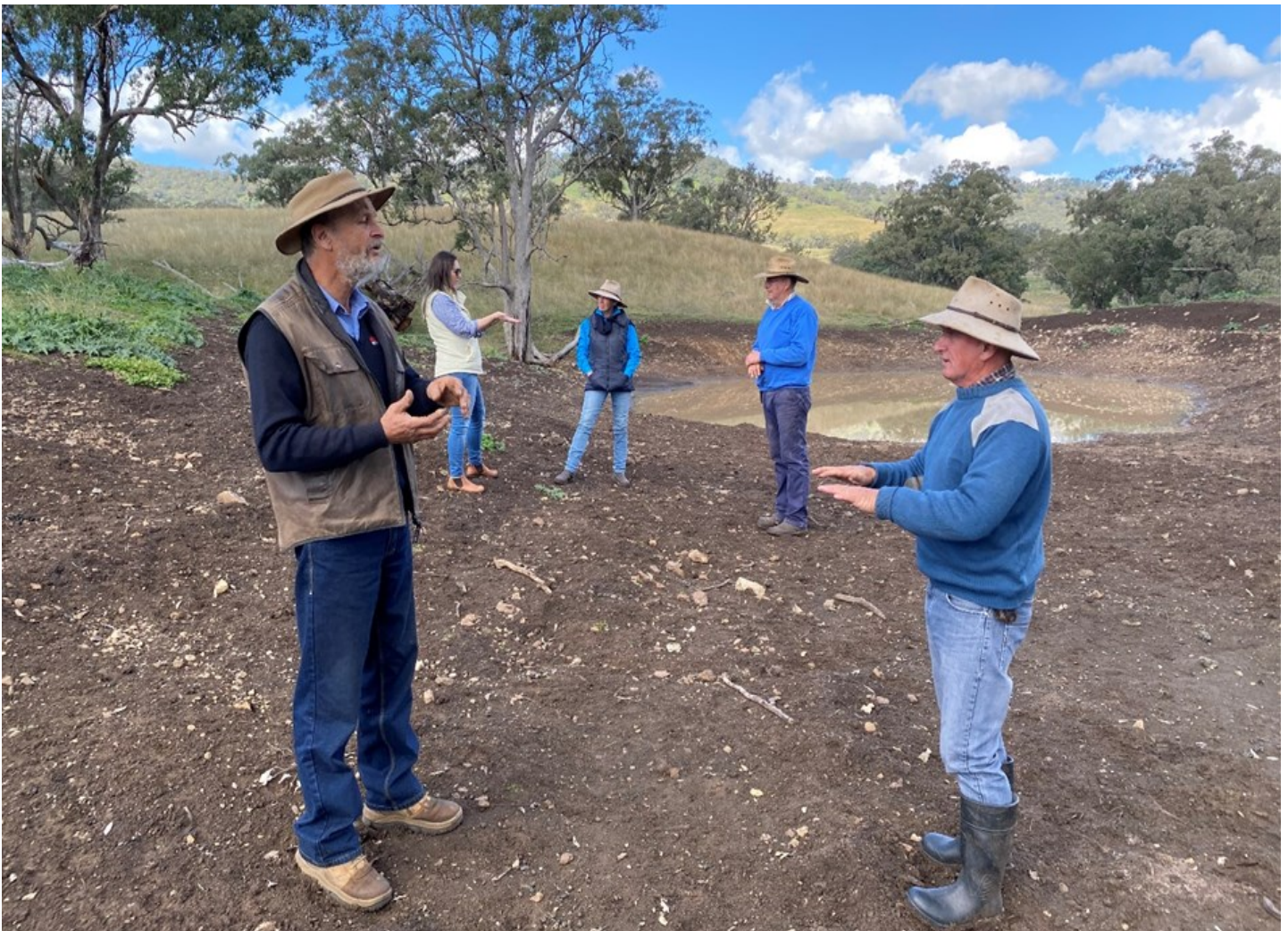
LLS Staff Tim Watts and Angela Baker discuss completed earthworks for Rehydration Project with UMLC’s Nicola Chirlian, Craig Carter and Myles Sevil at “Hillvue” McDonalds Creek.
